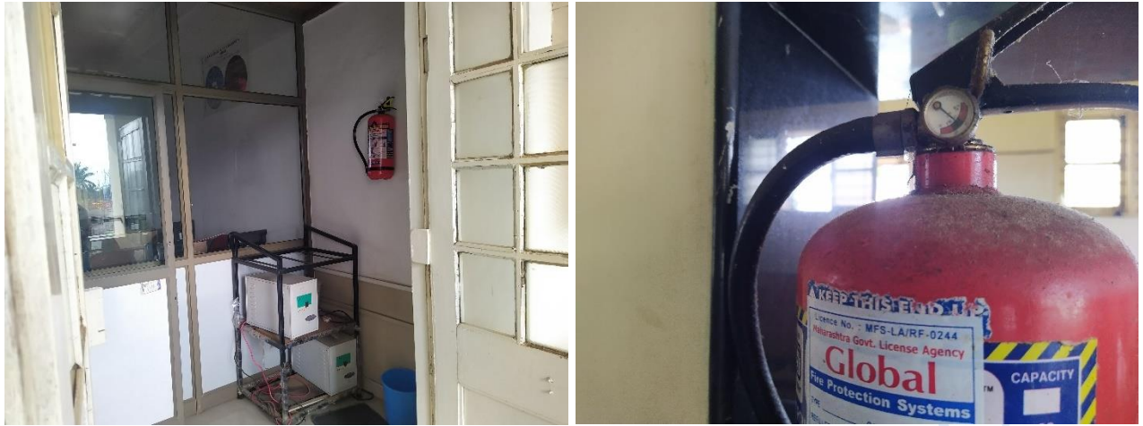
Figure 16 - No ready access to fire extinguisher.
