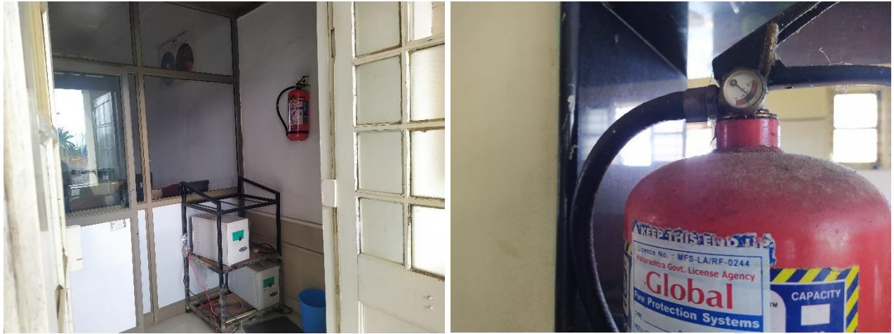
Figure 16 - No ready access to fire extinguisher.
