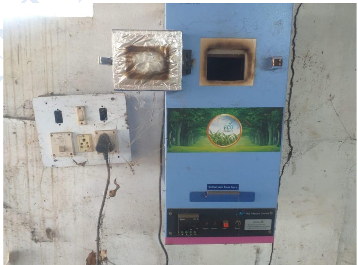
Figure 15 - No easy access to incenerator
