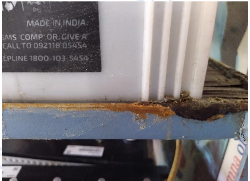
Figure 14 - Galvanic reaction : causes self discharging and degradation.
