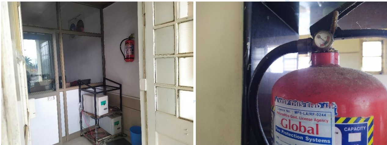
Figure 16 - No ready access to fire extinguisher.
