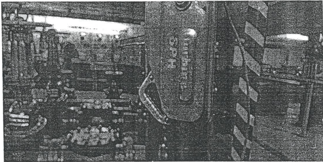
Seen are the shaft room and pumps for carrying coolant located at the minus one level
